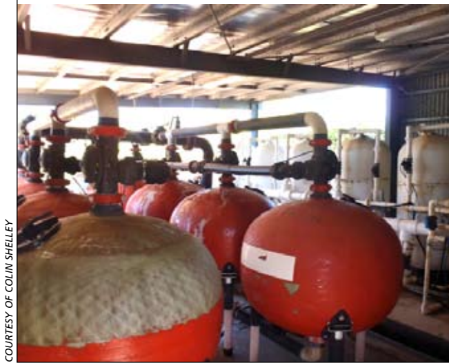
FIGURE 4.2 Bank of automated sand filters at the Darwin Aquaculture Centre
