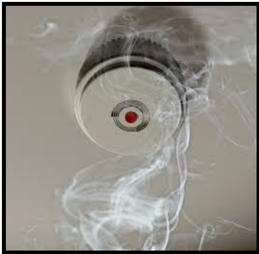
Figure 6-3: Automatic fire alarms.
