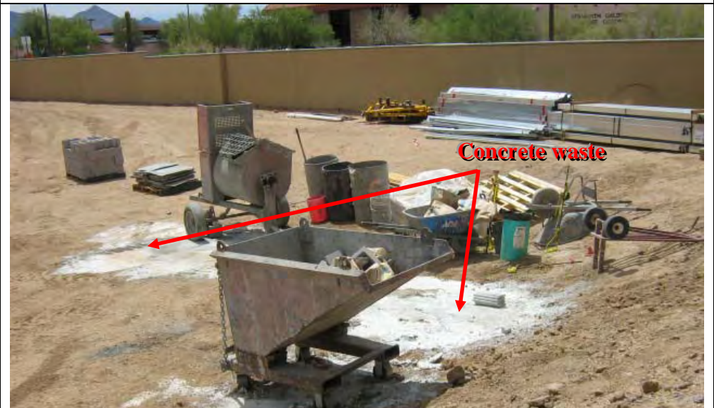
Photograph 4 – Potential source of the illicit discharge
