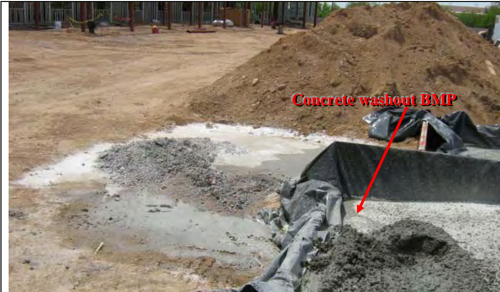
Photograph 5 – Concrete waste beyond the dedicated concrete washout BMP
