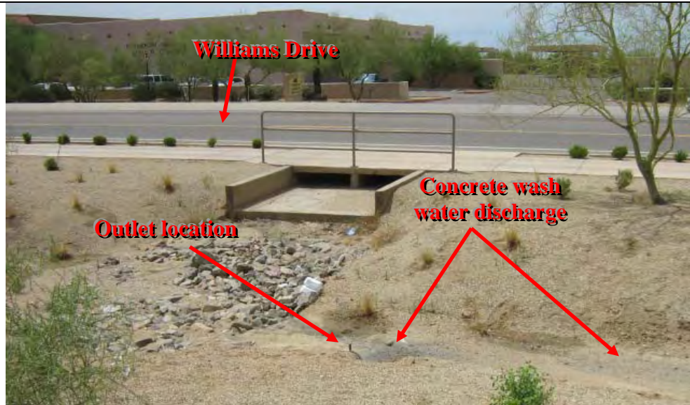
Photograph 1 – View of illicit discharge to a drainage ditch along Williams Drive
