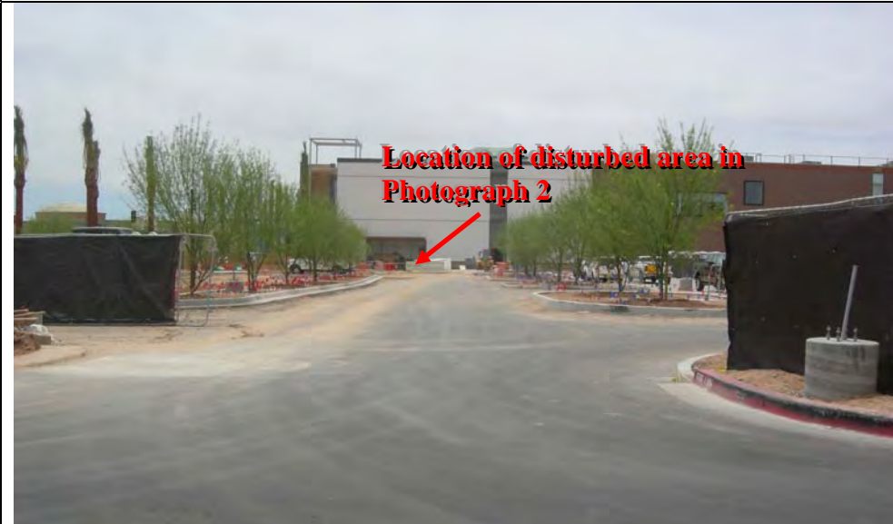
Photograph 3 - View of sediment tracking from the construction entrance at the northeast corner of the site, facing south.
