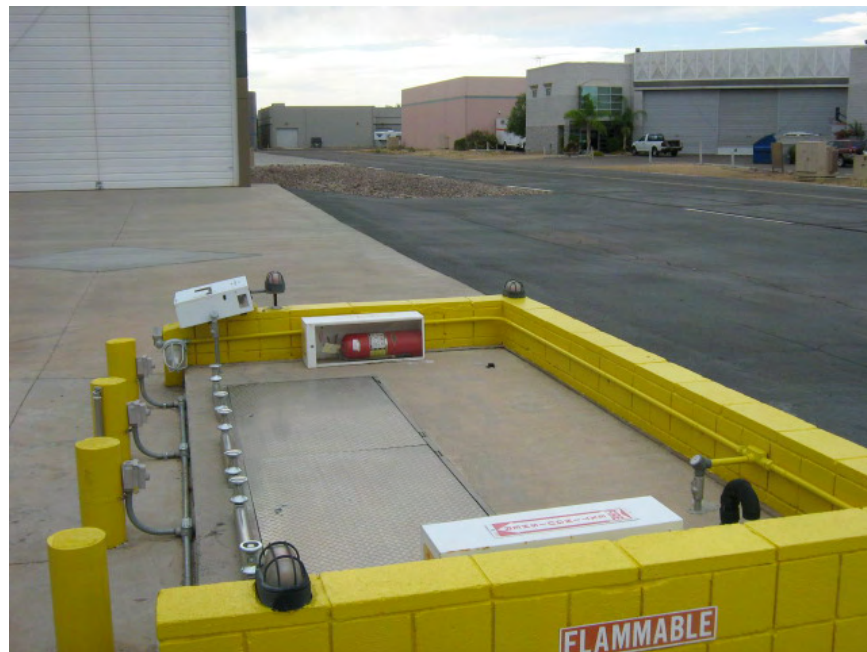
Photograph 4. Scottsdale Airpark – Aircraft fueling system located northeast of 7916 East Beck Lane in Scottsdale, Arizona
