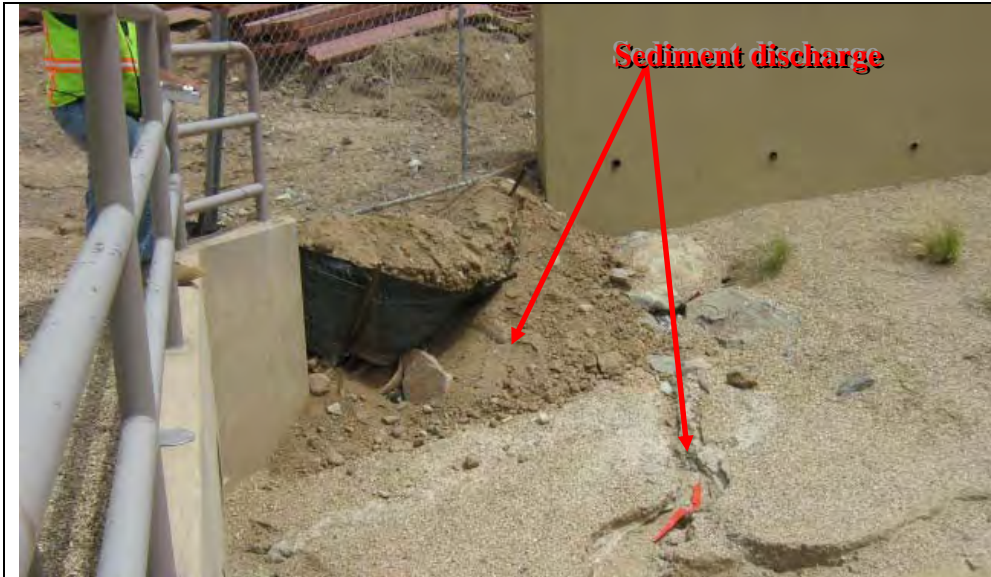
Photograph 9 – Silt fence failure and offsite sediment
