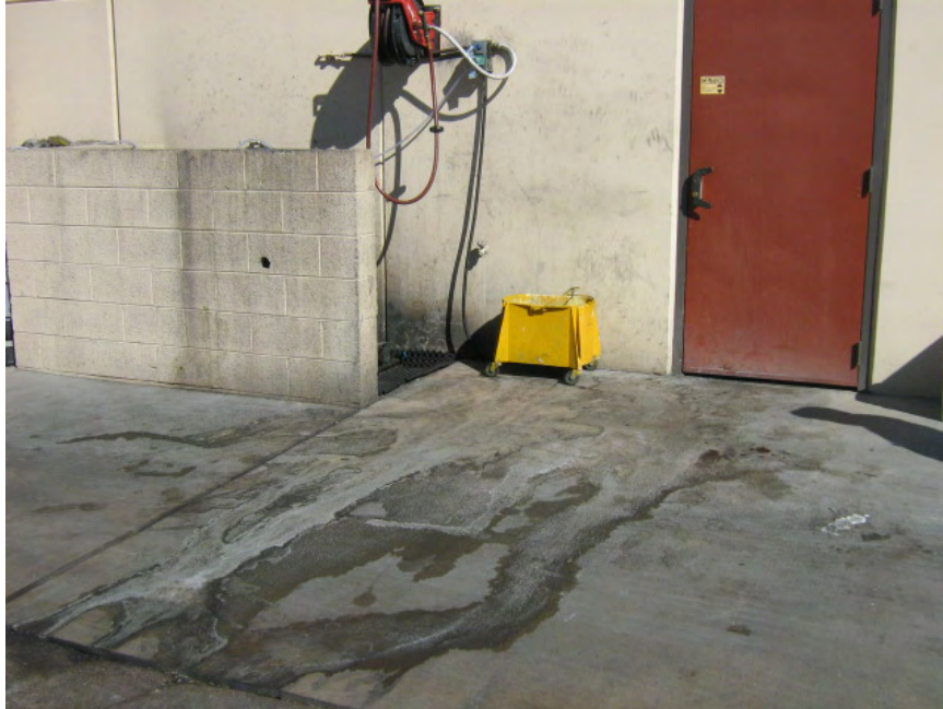
Photograph 9. Evidence of residue transport from designated degreasing area.
