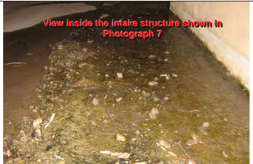
Photograph 8 – Sediment and debris accumulation in intake structure
