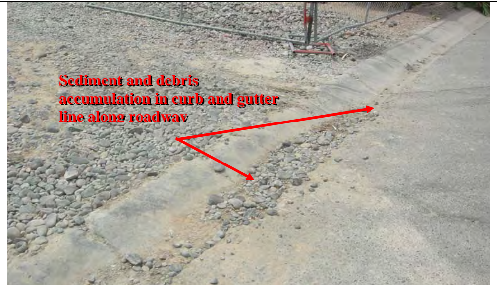
Photograph 4 – Sediment and debris accumulation at Phase II construction entrance
