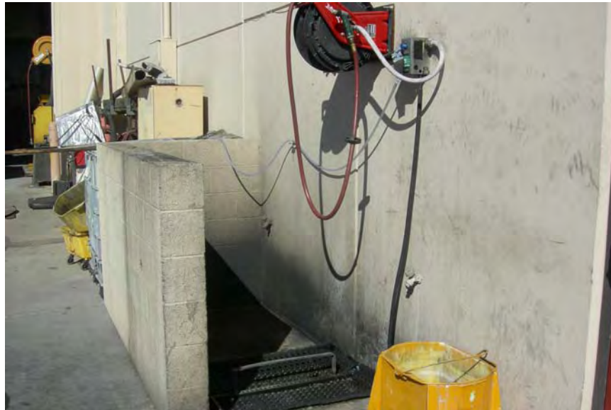
Photograph 8. Floor degreasing wash area located in the vehicle maintenance area of the North Corporate Yard.
