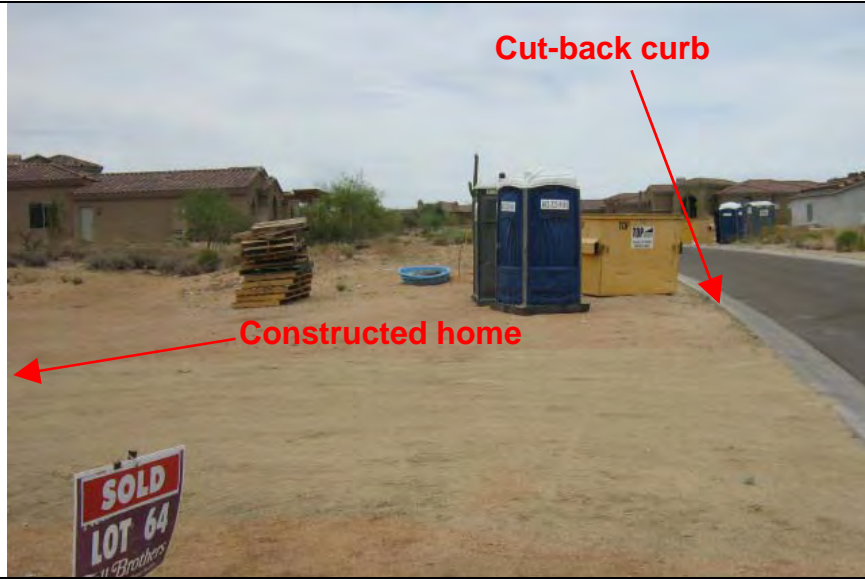
Photograph 3—Lack of perimeter control BMP
