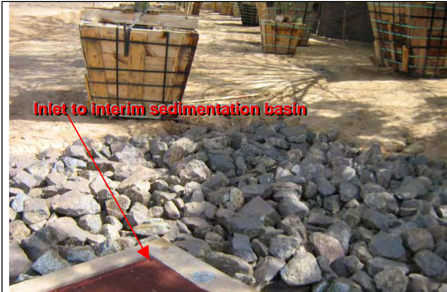
Photograph 5 – Irrigation activity located adjacent to interim sedimentation basin in the southeast portion of the site
