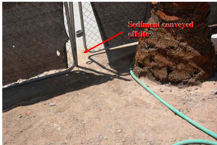
Photograph 6. View of sediment release along the east side of the Scottsdale Fashion Square construction site, adjacent to Scottsdale Road.
