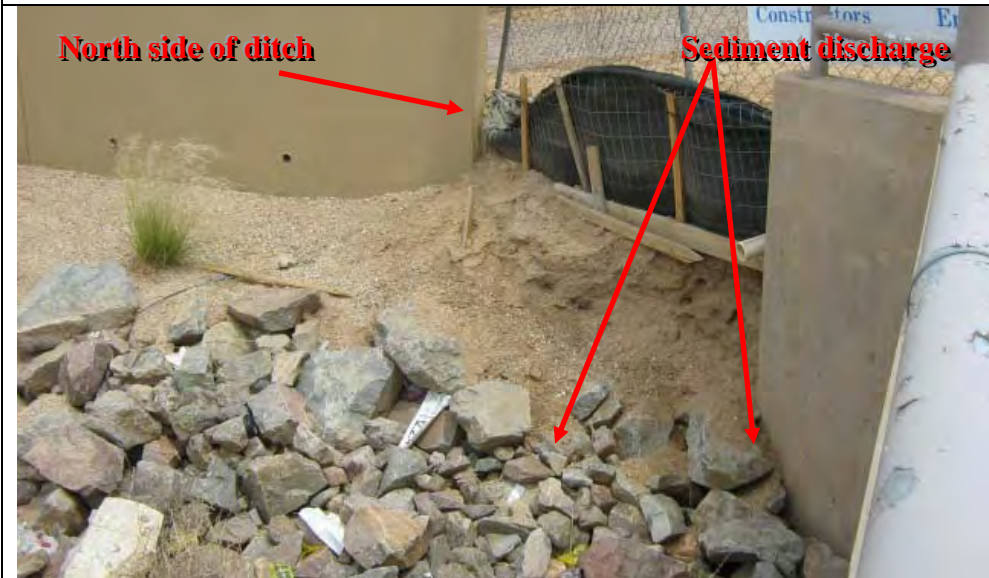
Photograph 7 – Silt fence failure and offsite sediment
