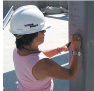
John Gardner '68 and Therese Gardner sign beams in the Walter K. Chess Center.
