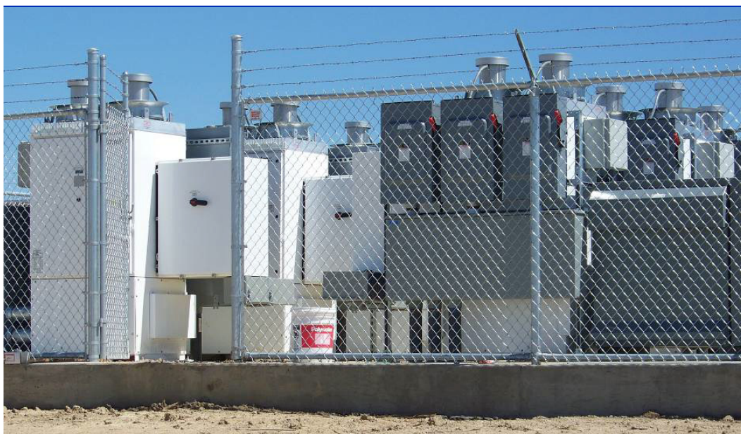
Figure 74. Utility-scale inverters use higher DC input and AC output voltages to reduce losses, and the size and costs of the conductors and switchgear required.
