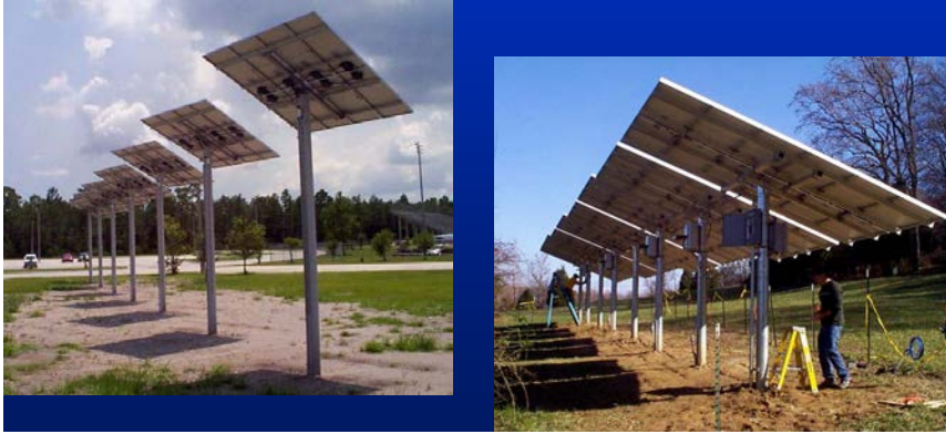
Figure 23. Pole-mounted arrays use either fixed, adjustable, or sun-tracking arrays installed on a rigid metal pipe.
