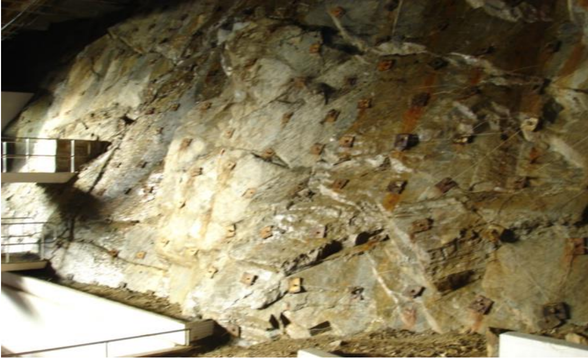
Figure 2.6: The cliff face formed the Aquadrome's fourth wall. Note the extensive bolting required to stabilise the cliff face (Photograph: Ricky Rooney and James Turpin)
