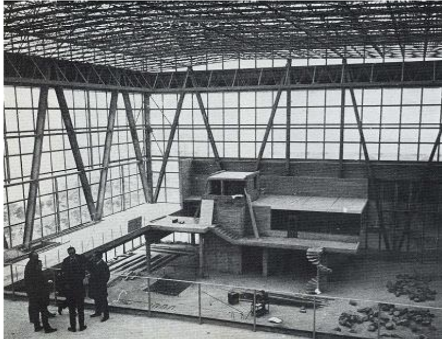
Figure 2.11: The shell of Summerland’s four upper floors. Much work remained to be done before the summer 1971 opening date. This photograph is looking down on the Solarium floor from one of the terraces. The building’s main entrance is in the left background.
