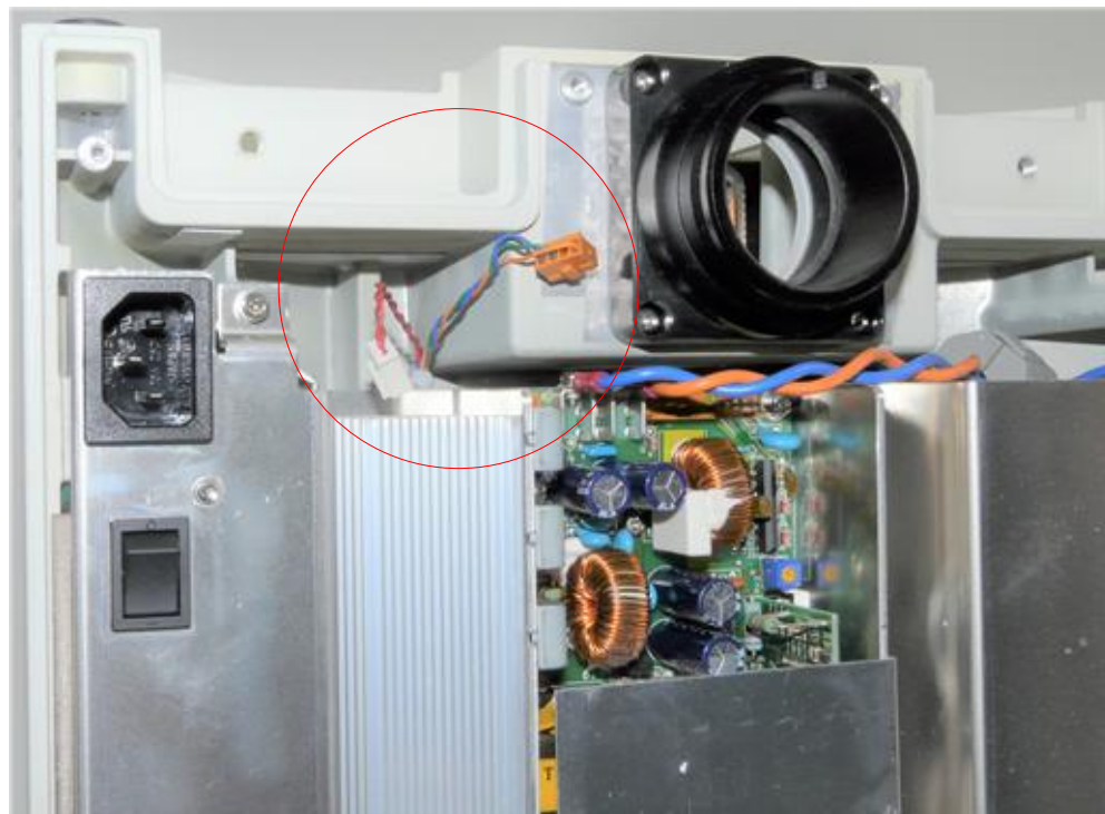
Photo 16. Disconnected cables (red circle).
