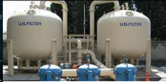
Tanks for an ion exchange perchlorate-removal process treat groundwater at a NASA-funded water plant.
