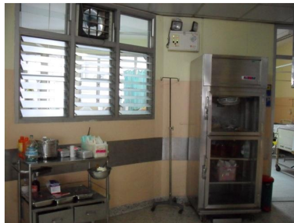
Fig. 10 Industrial type exhaust fan that was installed in the inpatient ward of hospital C
