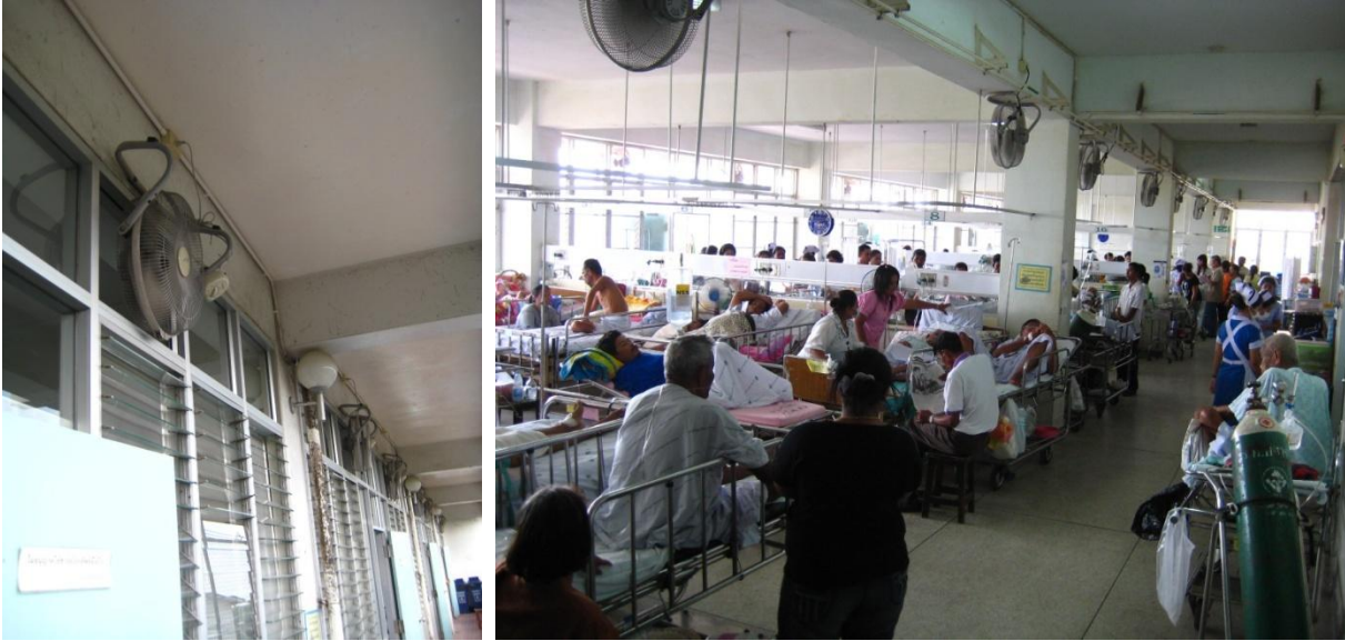
Fig. 11 Exhaust fans that were installed in the inpatient ward of hospital D
