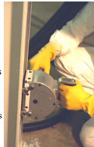
Figure 15: Shrouded Power Tools
