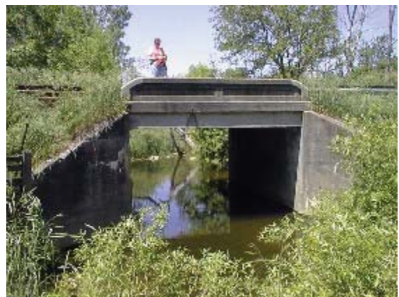
Figure 17: Field Crews Collect Information on Stormwater Retrofit Needs at MDOT Stream Crossings
