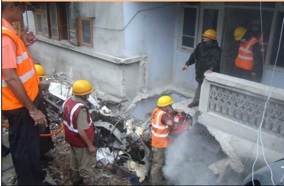
2 BN NDRF RESCUERS WORKING AT COLLAPSED BUILDING AT GANGTOK, SIKKIM
