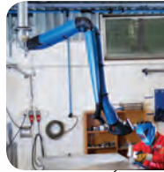
Extraction arm for welding
