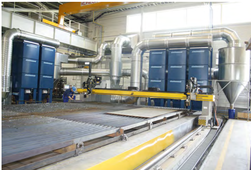
Fig. 2. CNC cutting table with a Nederman extraction installation.
