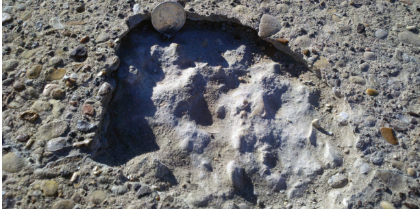
Hole in Concrete
