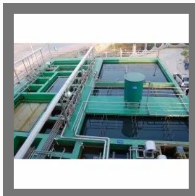
Industrial Sewage Treatment Plant
