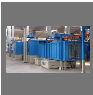
Industrial Pre Treatment Plant
