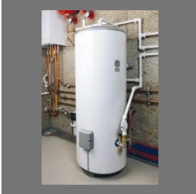
Hot Water Heater
