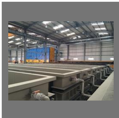
MS Pretreatment Tank
