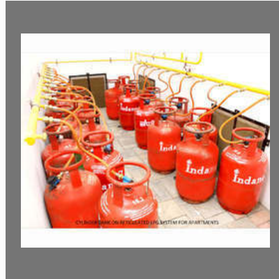
LPG Bank Installation Service
