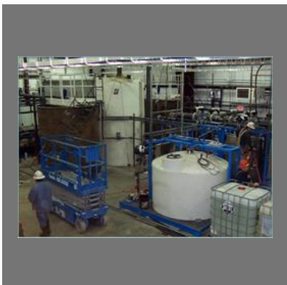
Water Filtration Plant
