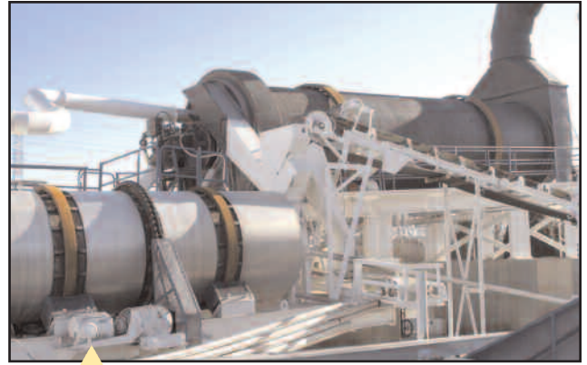
A secondary mixing drum that is used to blend the RAP and virgin components is shown on the left. The primary dryer is on the right.
