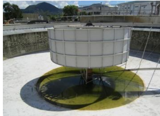
Figure 12 - Existing FCW design of Final Clarifier No. 2 at Tai Po Sewage Treatment Works.
