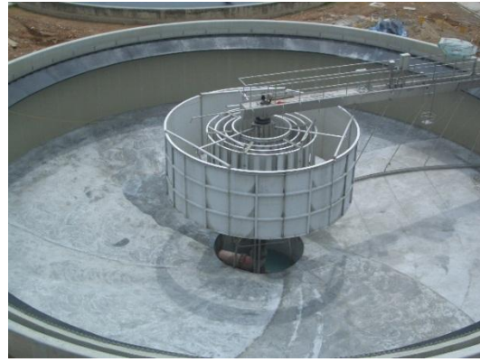
Figure 3 - General arrangement of existing flocculation centre well design (outside) and four layer of energy dissipating inlets at Tai Po Sewage Treatment Works.
