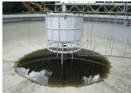
Figure 13 - New FCW design with FEDB of Final Clarifier No. 12 at Tai Po Sewage Treatment Works.
