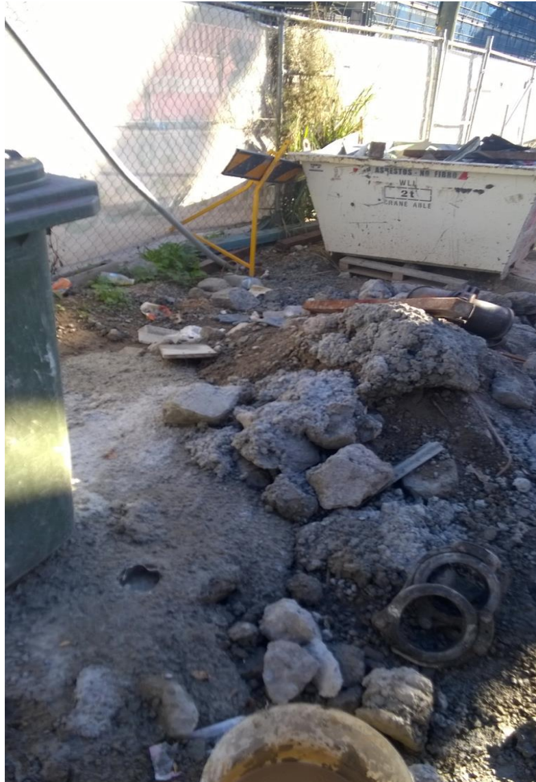
Figure 6. Lumps & material balls retrieved from grate of pump hopper
