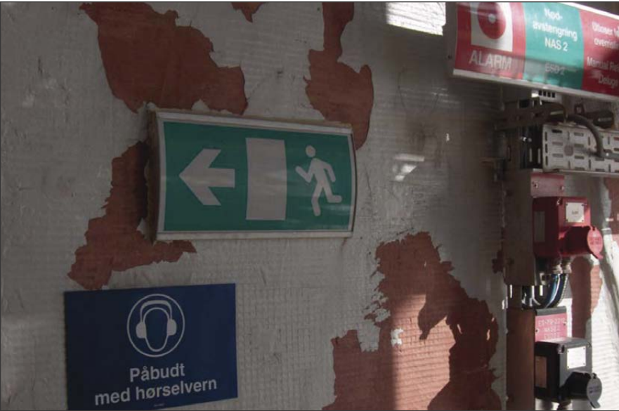
Fig. 1: Flaking observed on Grane, resulting most likely from a combination of the use of only a two-coat system and the properties of the paint applied. Problems with the adhesion and flexibility of the topcoat over time could have contributed to flaking.
