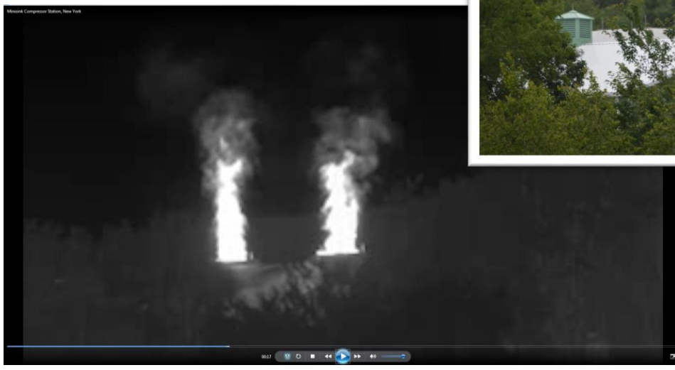
Emissions seen with optical gas imaging, Minisink Compressor Station, Orange County, New York. Images by Earthworks.
