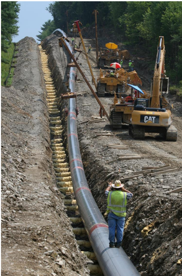
Forest cut for construction of the Millennium Pipeline, Broome County, New York. Photo by Roger Luther, nyslandmarks.com.
