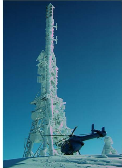
Figure 5-7: A broadcasting tower (continuing to function in ice / snow conditions)
