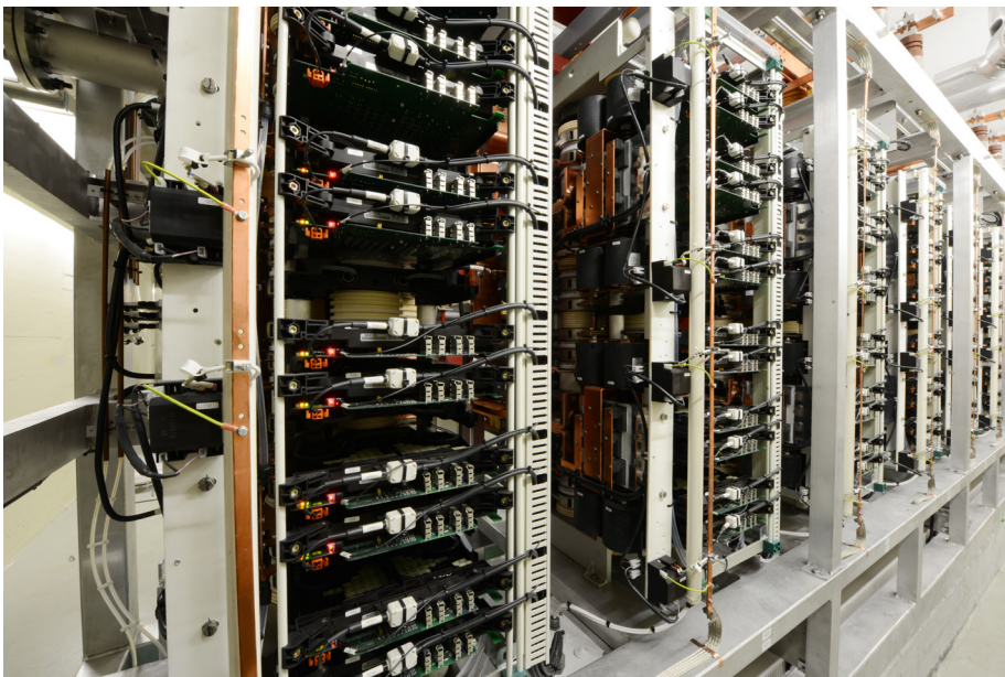
More than 1,000 IGCTs enable the pumped storage power plant Grimsel 2 to operate more flexibly and efficiently.
