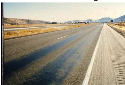
Slick 'bleeding' pavement
