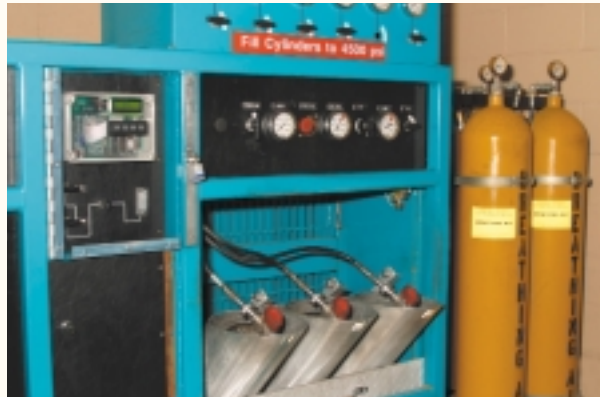
Figure 2-32 Air compressors are installed at many fire stations to refill SCBA cylinders.
