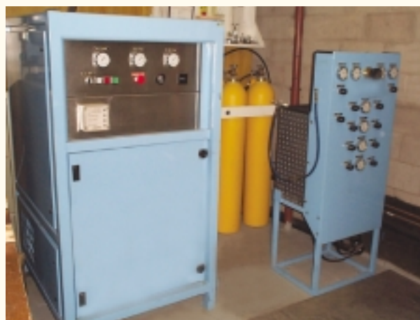
Figure 2-33 SCBA cylinders are refilled in a protective enclosure.
