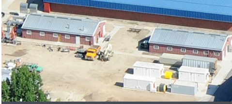
These two 1960s era ARMCO buildings were removed to clear the site for the new center.
