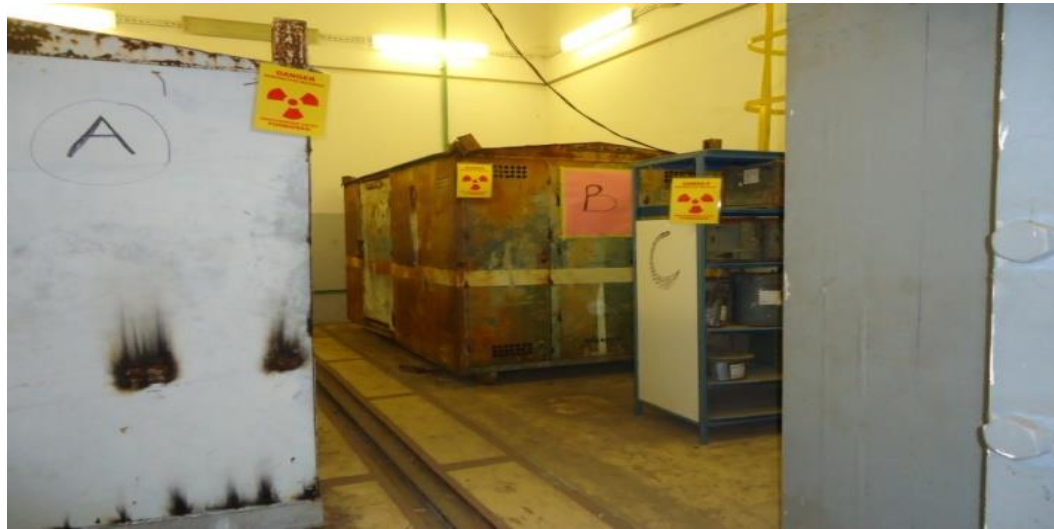
Plate 1: Temporary Storage at ASCL, Ajaokuta, Kogi State
