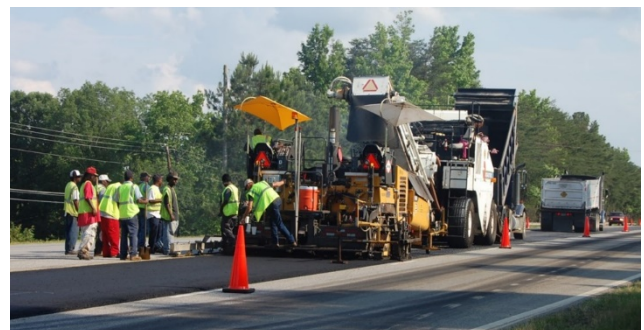
Thin asphalt overlays can be placed with conventional paving equipment for a quick, efficient operation.
