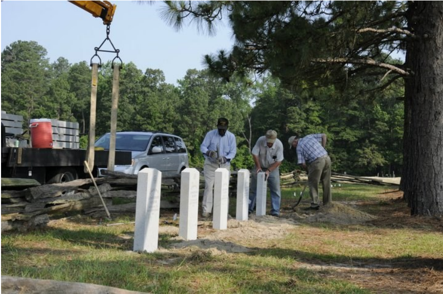
Figure 10. Unknown Confederate Soldier grave markers were installed over the measured locations of the 20 identified burial pits on June 8, 2011.
