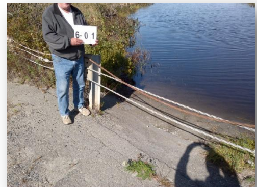
Road shoulder erosion near the boat launch in Sector 6.
