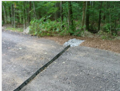
Reshape gravel roads, and add new surface material and install runoff diverters
