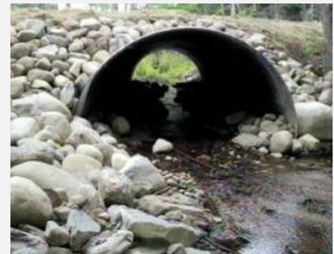
Replace undersized and perched culverts, remove clogs, armor inlet/outlet and install plunge pools
