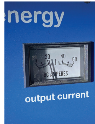
Charger (indicating 20A output)
