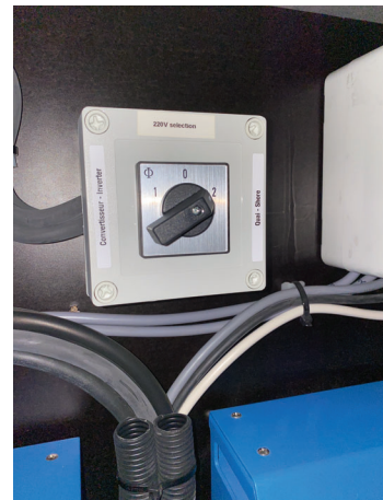
220v selector (showing shore power position)
