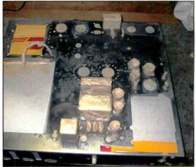
Photo H: Here's how the main chassis looked after rust was removed and all traces of the naval jelly were thoroughly washed away. Note that while the chassis now shines, blotchy areas remain where the rust has eaten through the factory plating. An unfortunate side effect was the loss of the factory decals for the tube types and alignment points.
