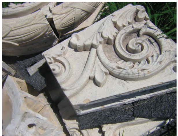
Opposite page: Phase I Rehabilitation, 2004. Top: The demonstration wall constructed in 2004 as part of Phase 1 to illustrate the method used to repair the exterior brick veneer, (photo taken 2019). Bottom: Example of the terra cotta detailing, much of which has been stored in the building.
