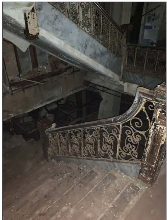
Original interior features, such as the grand stairs, must be retained and repaired to the greatest extent possible.
