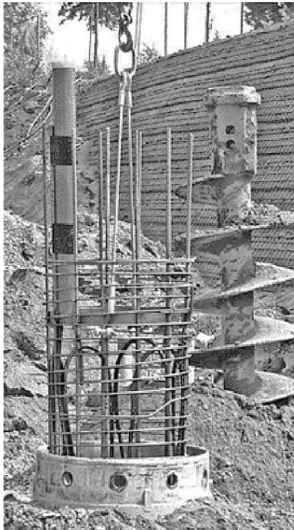
Figure 5: large diameter auger pile with reinforcement cage and heat exchanger loops inserted, the auger is in the background.
