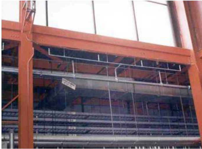
Figure C.9: Example of Cable Trays in Turbine Hall
