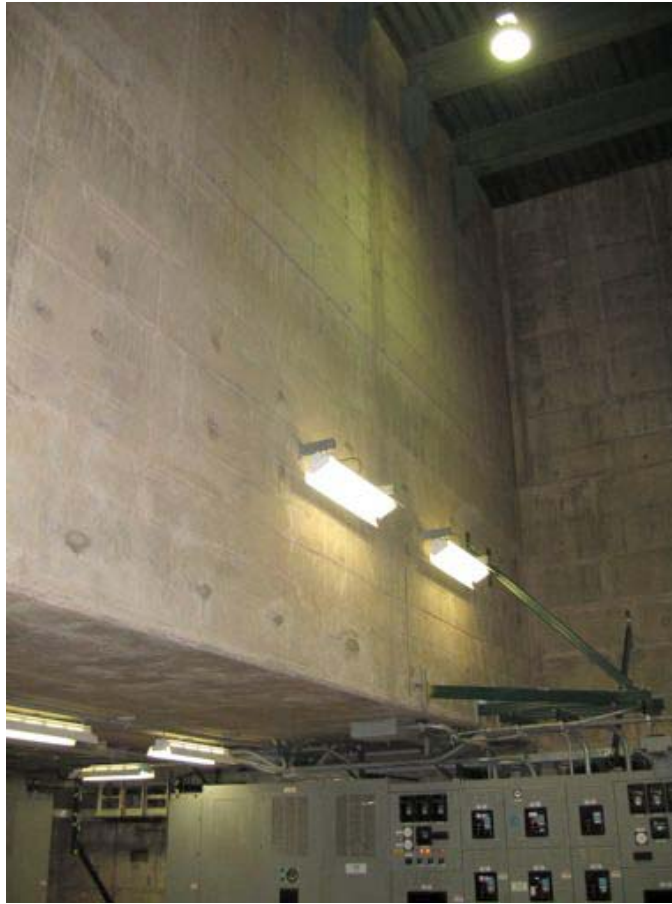
Figure B.2: Example of a Switchgear Room
