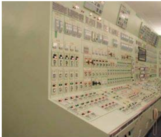
Figure A.5: Example of an Analog Control Panel in a Main Control Room
