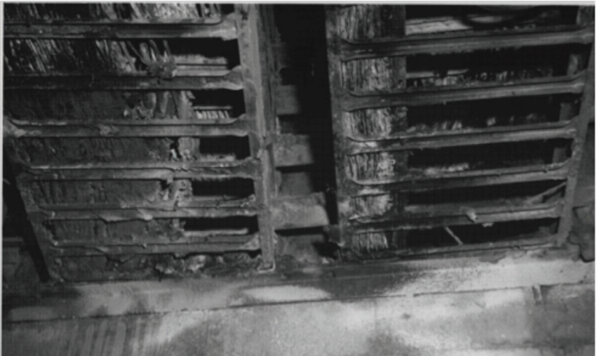
The Browns Ferry (BFN) cable tray penetration after the 1975 fire. The fire forever changed how the NRC and industry view the threat of fire (NUREG/KM-0002).
