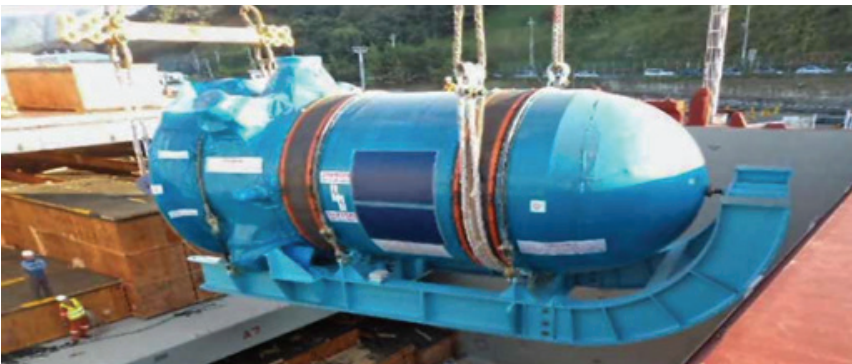
Vogtle Unit 3 (AP1000) nuclear island; rebar placement in preparation for concrete basemat pour (Top). Vogtle Unit 3 reactor pressure vessel arrives in the United States (Bottom). Courtesy of Georgia Power, a Southern Company.
