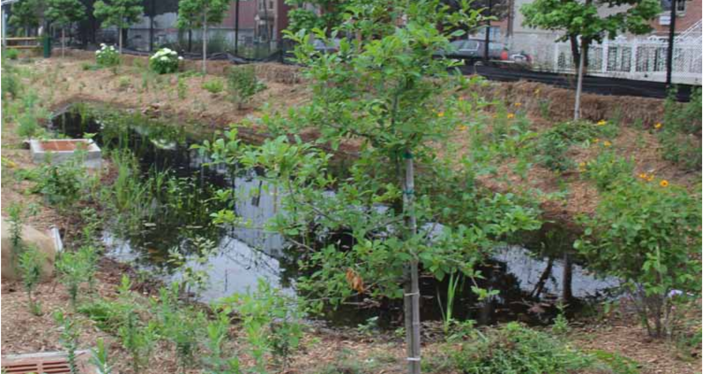
In May 2011, DEP constructed a pilot mini-wetland and bioswale system in the parking lot of an MTA bus depot in Brooklyn.
