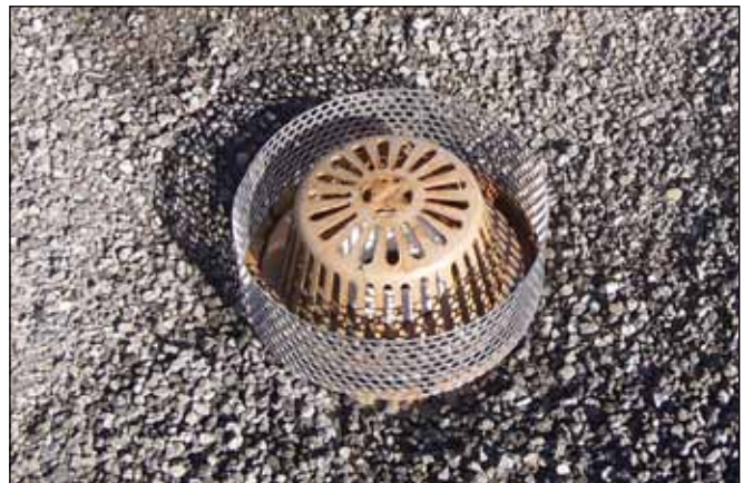
DEP installed a modified drain cover in the second quadrant to control the flow of stormwater off the roof.
