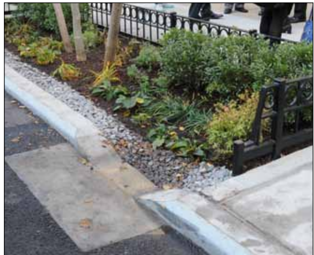
After evaluation of the first generation of inlets, DEP replaced some of the inlets with depressed curbs to increase stormwater conveyance into the ETP or SSIS.
