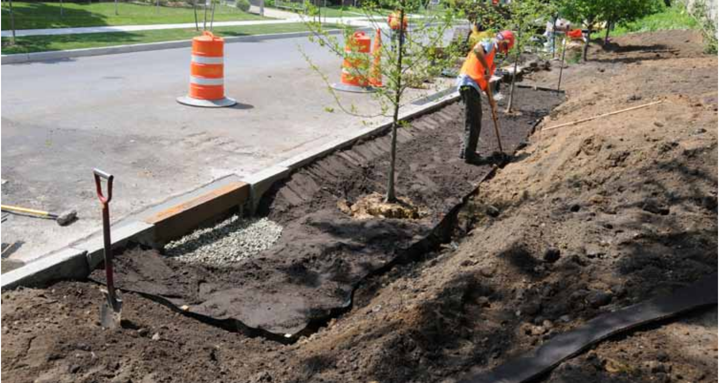
Streetside infiltration swales, such as this one located in Brooklyn, can manage thousands of gallons of stormwater each year.
