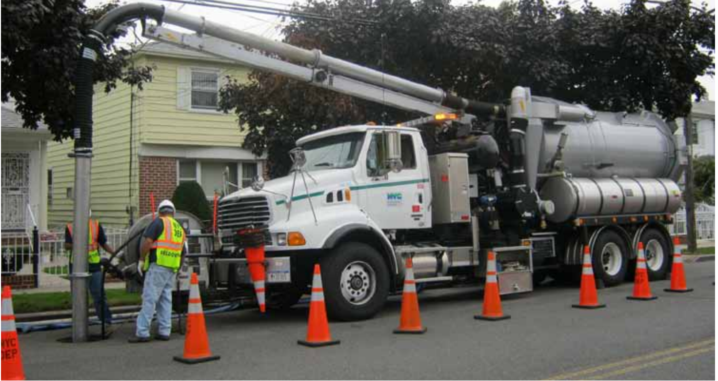
DEP uses Vactor trucks to remove sedimentation from the sewer system, increasing its capacity to hold wastewater during wet weather.
