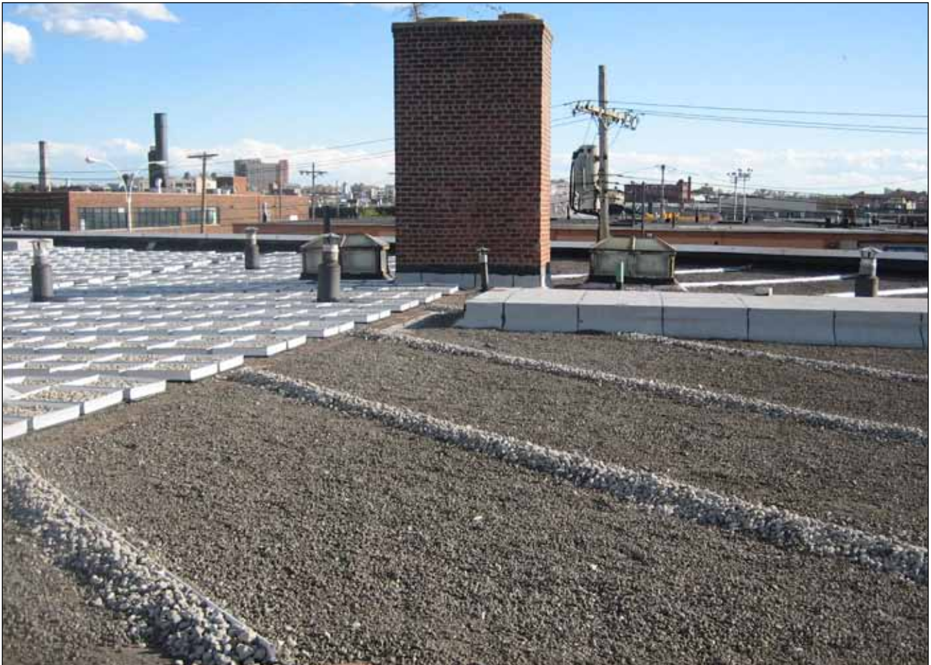
DEP piloted three different blue roof technologies on the rooftop of one of our general storehouse facilities in Brooklyn. The design includes a tray and ballast system, on the left side of the above image, and an intermediate check dams system, on the right side of the image.
