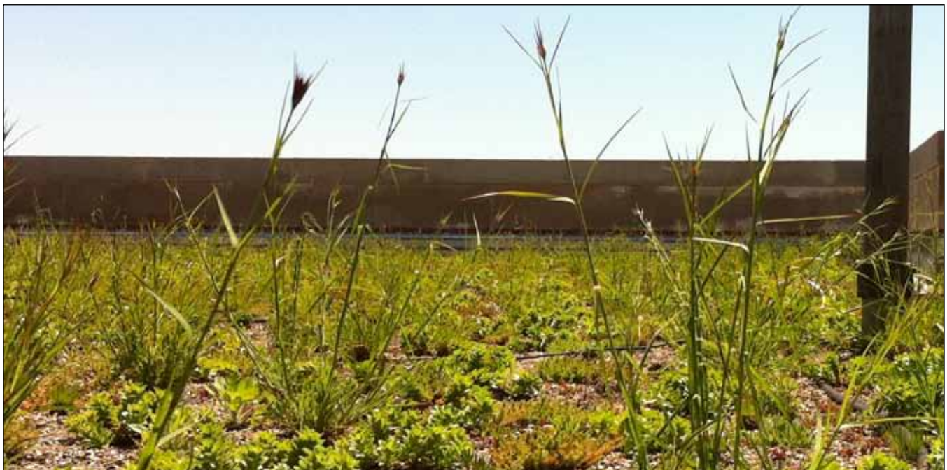
Green roofs are designed to absorb rainwater until it can evaporate or be consumed by the vegetation through evapotranspiration.
