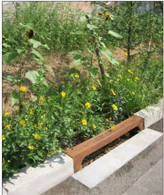
SSISs are 40 feet long, five feet wide, and 4.5 feet deep, and have only one subsurface layer made of engineered soil.
