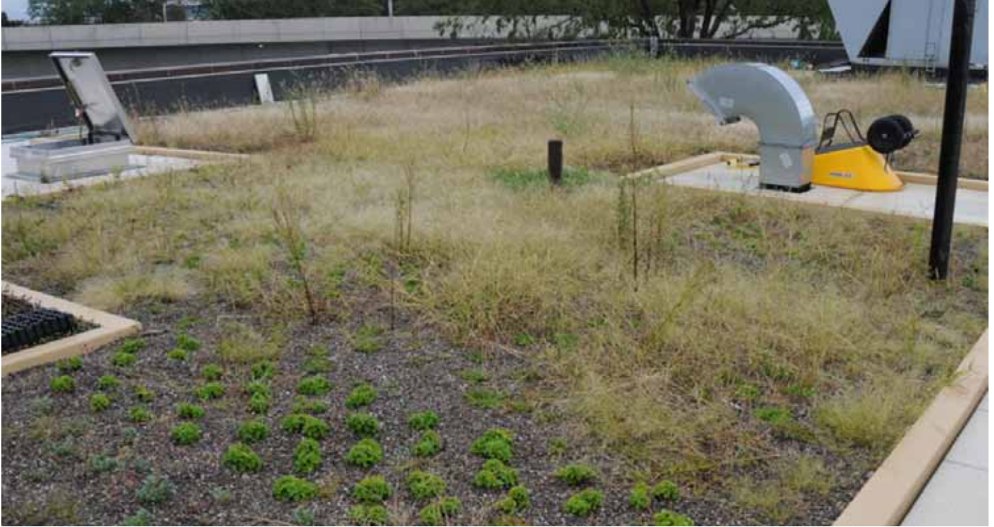
The Jamaica Wastewater Treatment Plant green roof manages more than 13,000 gallons of stormwater each year, reduces the building's absorption of ultraviolet light, and improves insulation.
