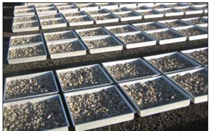
DEP installed a tray and ballast system in the fourth quadrant that detains stormwater in 1,600 trays before it eventually drains off the roof.
