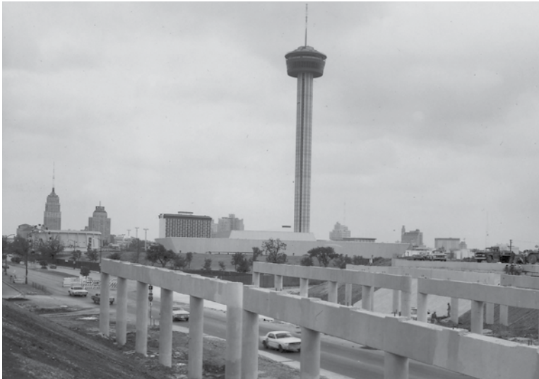
Construction I-37 at Durango Boulevard in San Antonio, Photo courtesy TxDOT Library
