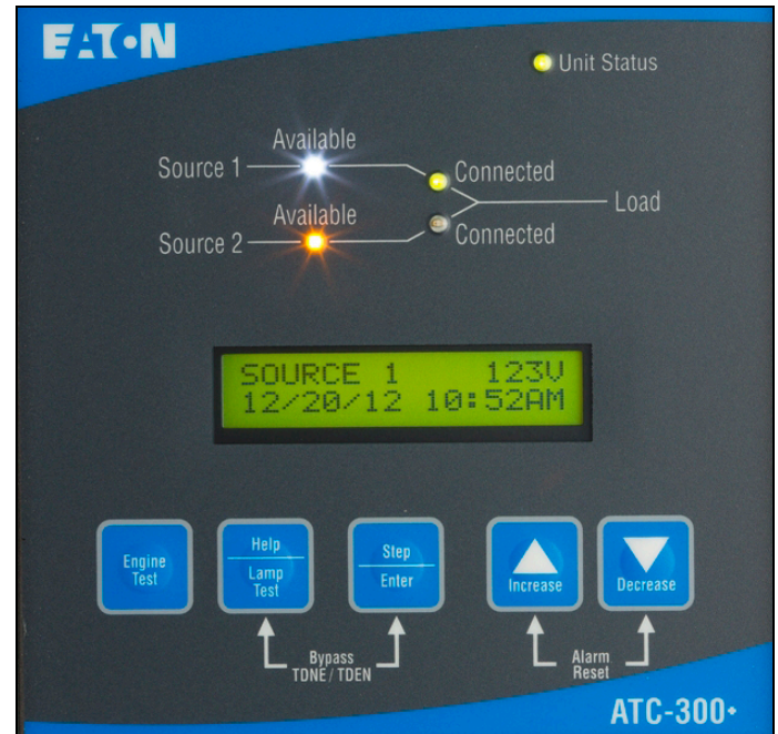
Figure 7. ATC-300+ Logic Control Panel.
