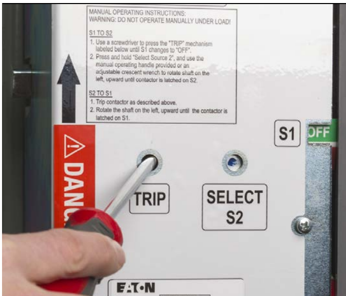
Figure 12. Trip Button on Contactor Operating Mechanism.
