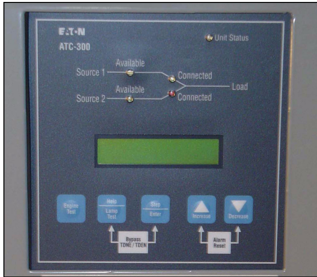
Figure 1. The ATC-300 Controller Front Panel.
