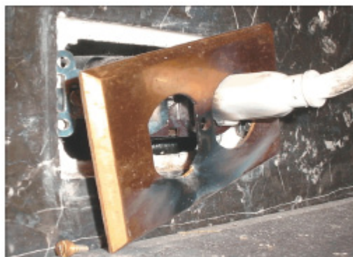
Figure 5. Electrical outlet without a cover
