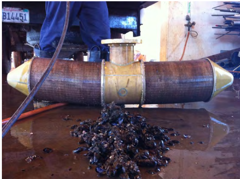
Mussels Removed from the Cook Legacy Screen after Failure
