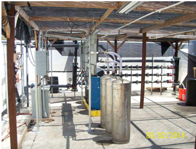
Intake Pipe Testing Facility
