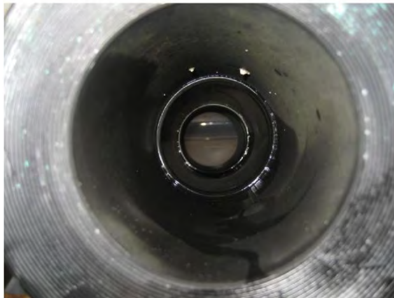
Figure 3-6. Pipe spool C4 (Shock Chlorination) December 23, 2014. Inlet (top) and Outlet (bottom).
