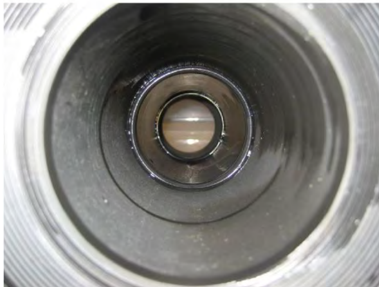
Figure 3-5. Pipe spool B4 (Continuous Chloramine Injection) December 23, 2014. Inlet (top) and Outlet (bottom).
