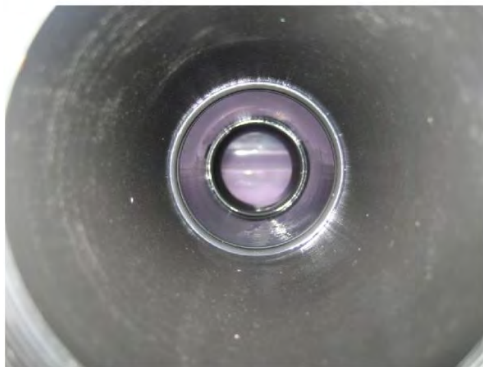
Figure 3-2. Pipe spool B3 (Continuous Chloramine Injection) October 28, 2014. Inlet (top) and Outlet (bottom).
