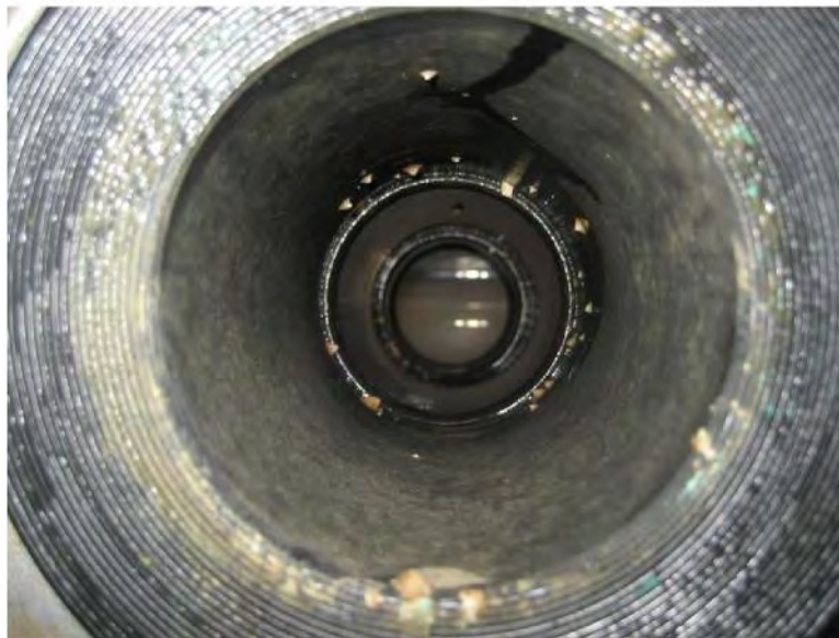
Figure 3-4. Pipe spool A4 (Control) December 23, 2014. Inlet (top) and Outlet (bottom).
