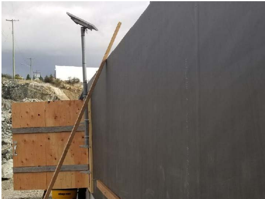
Photo 2 – Solar Panel Installed and Operational at Leachate Storage Facility.
