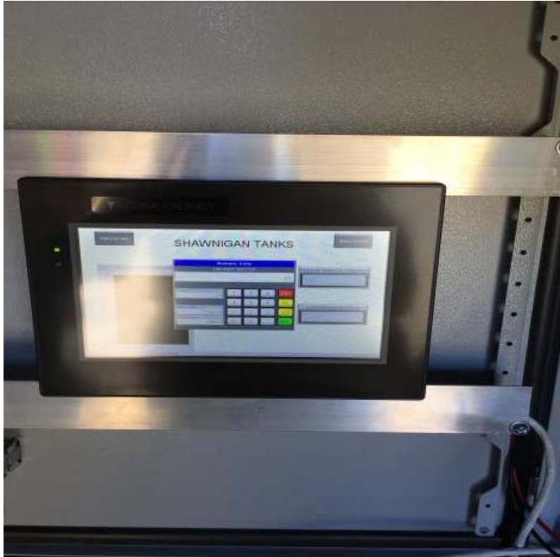
Photo 3 – Digital Readout Screen on Inside Door of Control Panel – for High-level Alarm.
