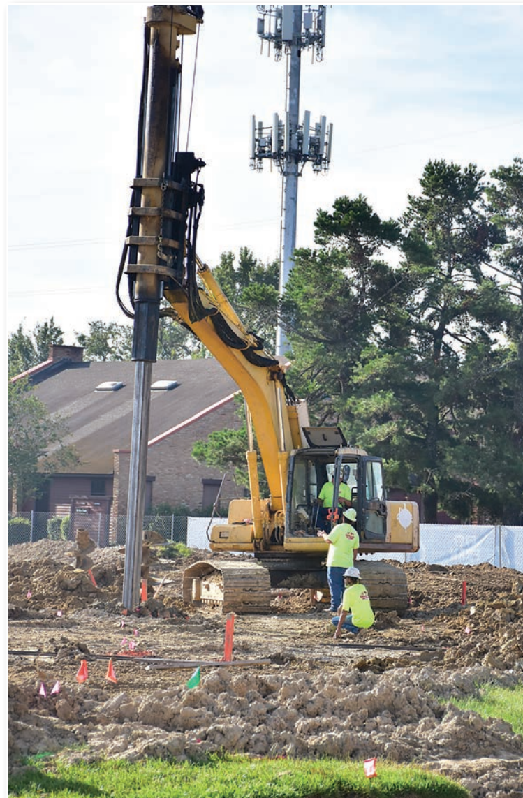
Workers are on site using heavy equipment to take soil samples and other work.
