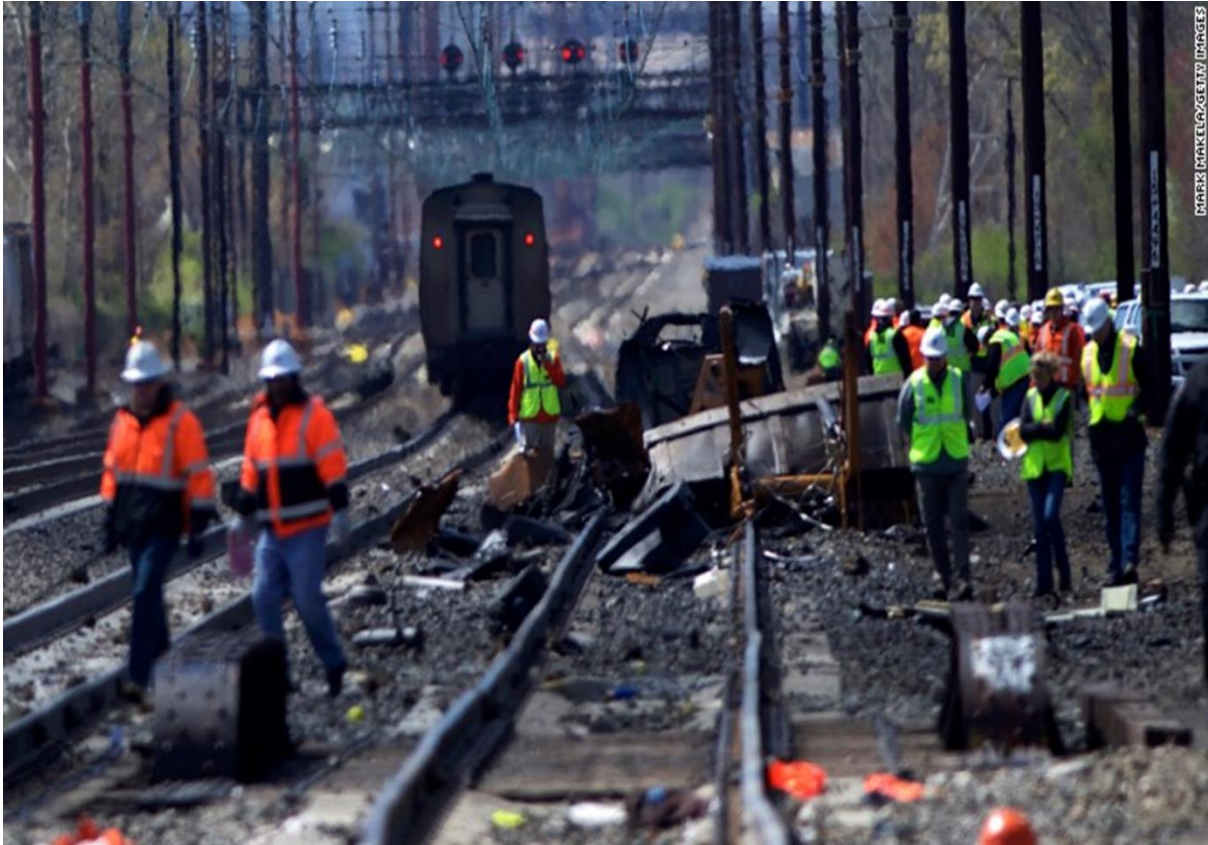
Figure 2: Last Amtrak 89 Collision Site
