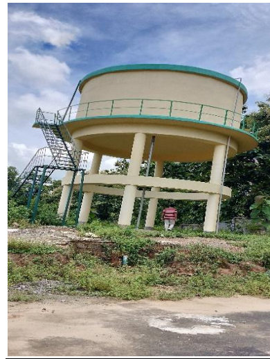
Overhead Water tank
