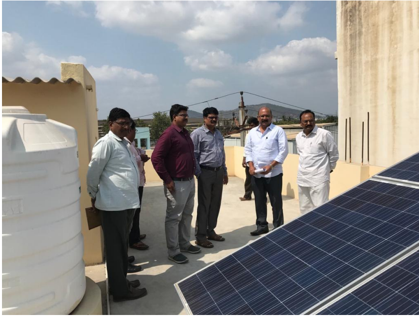
Solar Panels installed on Common Facilities Centre Building at JRD Tata Industrial Estate
