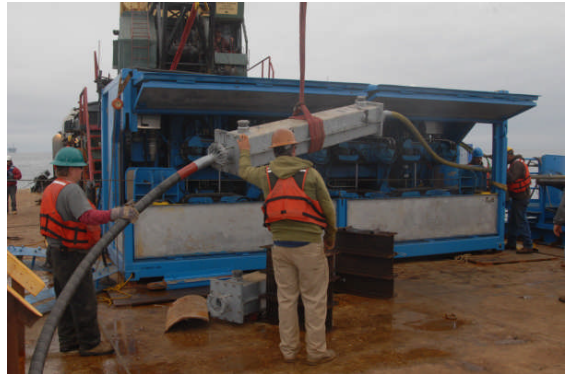
Figure A.8: Splice box rigged and ready
