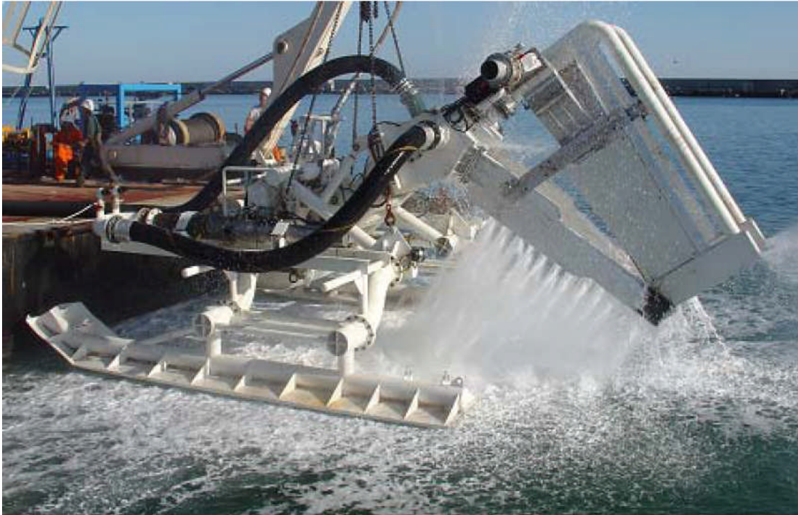
Figure 9.6: Cable Jetting device. The sword carrying water nozzles is visible and working. (Courtesy of L D Travocean, France)
