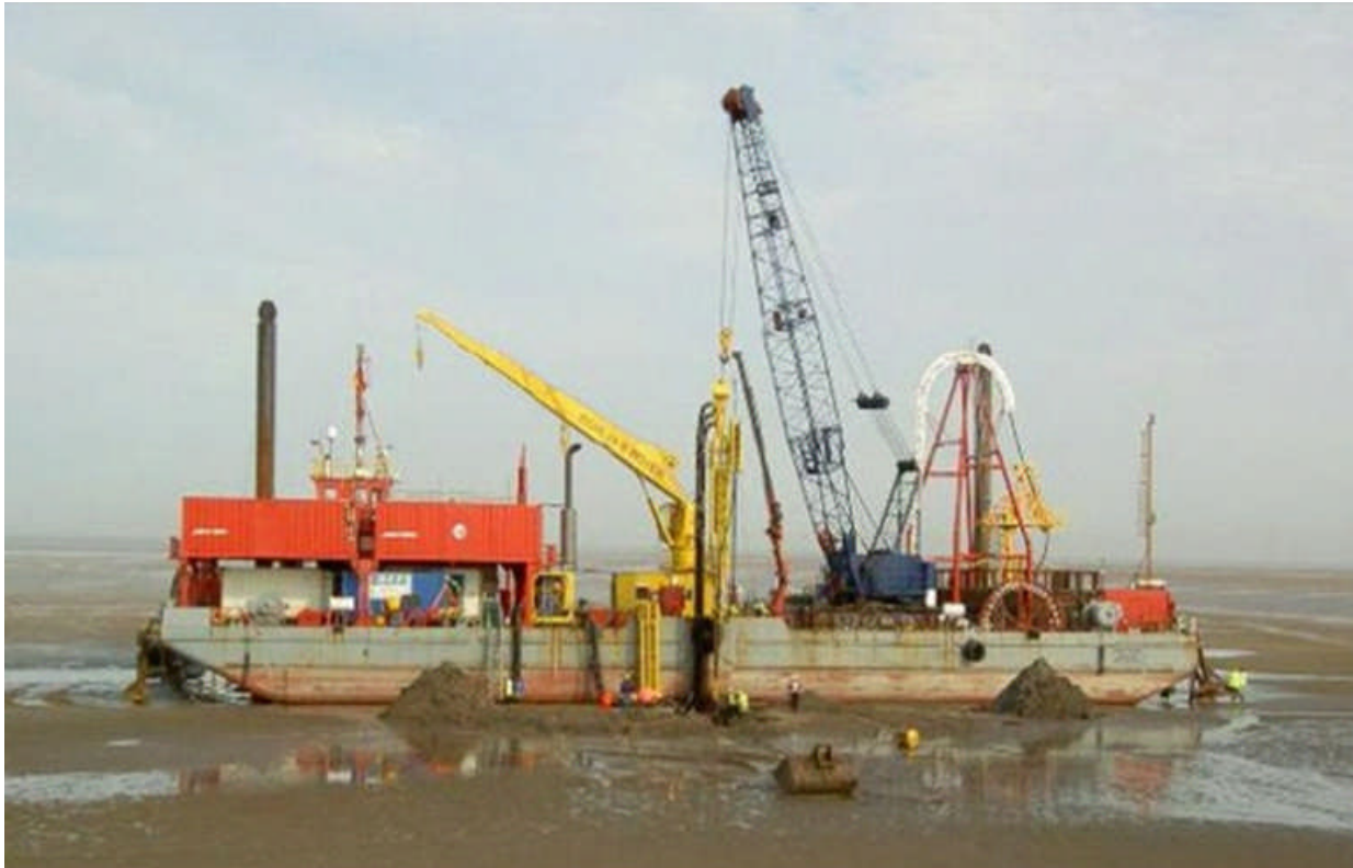
Figure D.1: Oceanteam Installer – a flat bottom barge (Courtesy of Oceanteam Power and Umbilicals).
