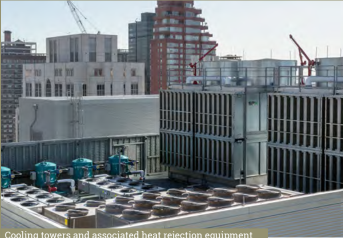
Cooling towers and associated heat rejection equipment
