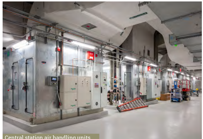
Central station air handling units
