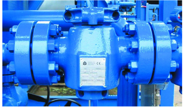
PLUG VALVE INSTALLED IN A SAND FILTER SYSTEM
