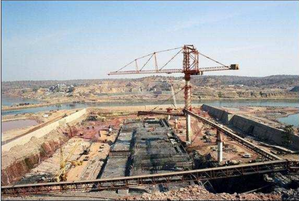
Fig. 24: The Omkareshvara dam in the course of construction (southern part); on the opposite bank, the power station. Source: CREMIN Emilie, March 2005.
