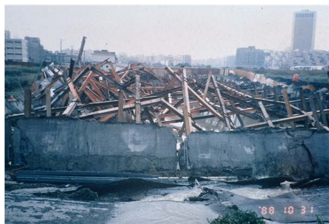
Fig. 1 Excavation failure in soft clay, Taipei, 1988
