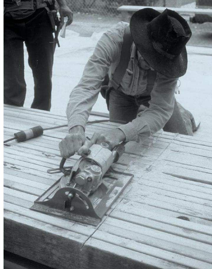
One at a time takes too long. The demand for housing was so great in the 1950s that tract builders used every trick they could to build faster and more efficiently. Cutting multiples was a common theme. Here, an entire roof's worth of rafters has been ganged up, and Larry is cutting the bird's mouths using a worm-drive saw with a swing table.
